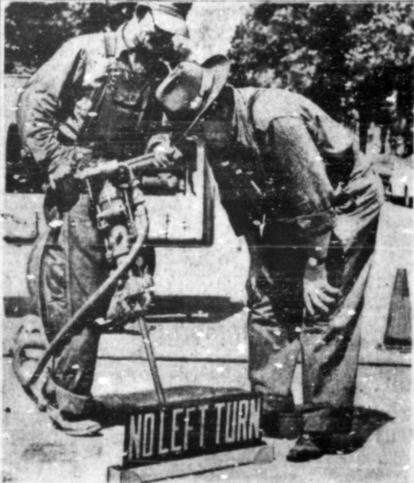
RUBBER TRAFFIC SIGNS advising of a prohibition on left turns were being placed at four intersections today by city crews. The 24x8-inch signs, with yellow letters, were set at 45-degree angles in the middle of the intersections, to be directly in line of vision of a driver starting to turn left. They were placed at Armour and Troost, Armour and Main, Linwood and Troost and Thirty-ninth and Main. William C. Puckett, an employee of the traffic engineer's department, prepares to operate a pneumatic hammer while N. L. Tullis, superintendent of street marking, views the marker, with its steel base, which will be sunk in the pavement.—(Kansas City Star photograph).
